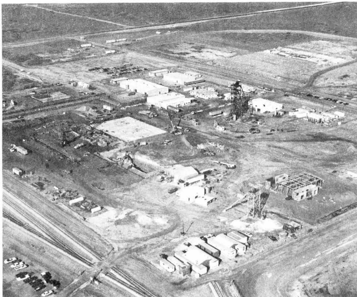
AERIAL PHOTO of the WIPP site shows surface facilities under construction. Tower at center right is the head frame over the personnel and salt-handling shaft that extends down some 2150 feet to a complex of tunnels and chambers in a geologic formation of salt, the future destination of radioactive waste.
